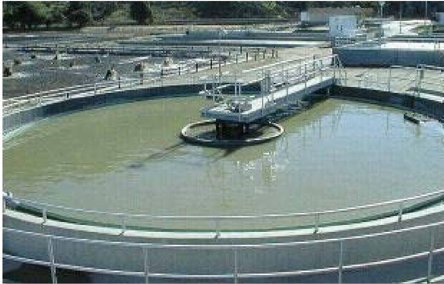
Figure 5: Primary clarifier ( http://www.ci.camarillo.ca.us/i3.aspx?p=1047 )
