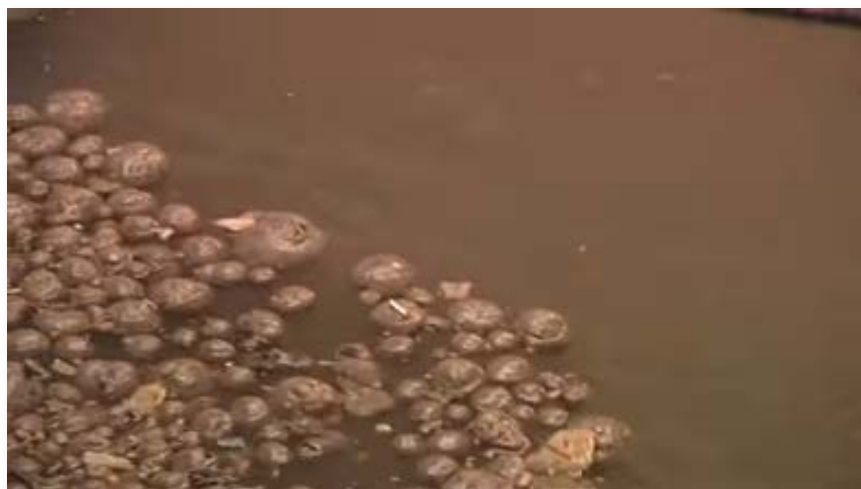
Figure 6: Grease balls forming in the wet well ( https://www.youtube.com/watch?v=pRaptzcp9G4 ).
