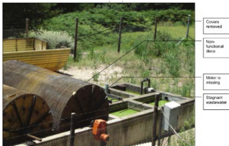
Figure 10: Poorly maintained rotating biological contactors (SOURCE: Boyd & Mbelu, 2009)
