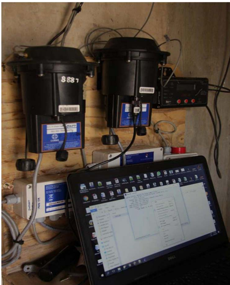
Figure 14: Capacity development includes the application of improved systems and infrastructure that can enable the system to function more efficiently. The image shows the water quality and quantity tracking system installed by RESILIM O along the lower Olifants River.
