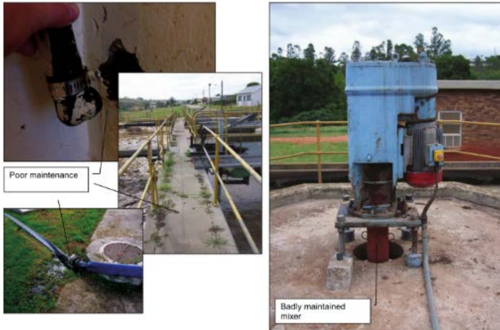
Figure 17: Example of bad maintenance (SOURCE: Boyd and Mbelu (2009), pg. 69)
